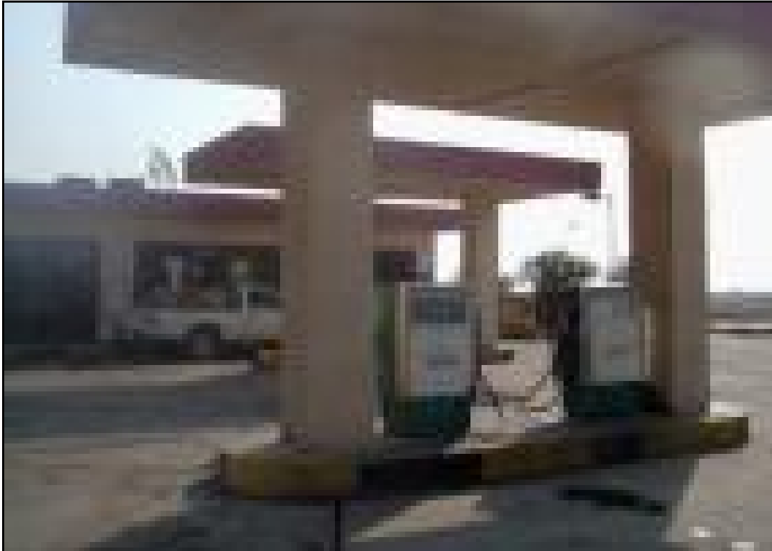
View of dispensers and island.
