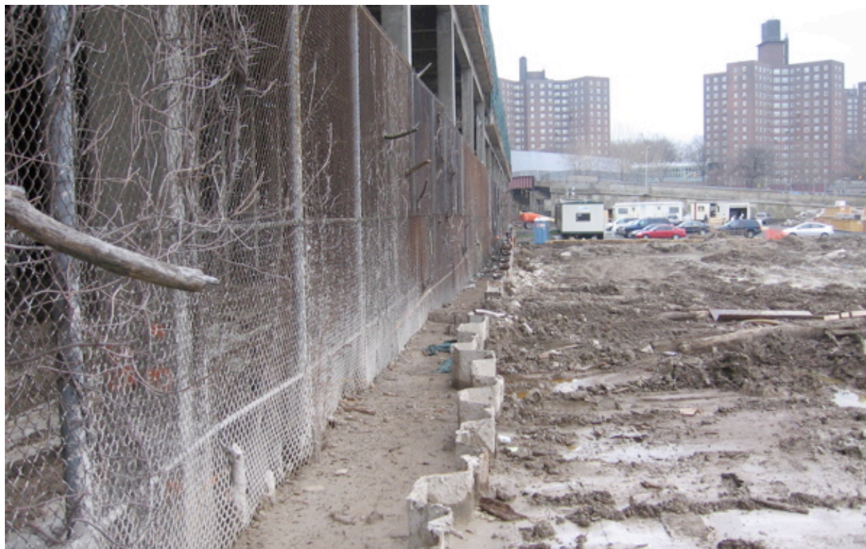
Waterloo® Barrier (along center of photo)
